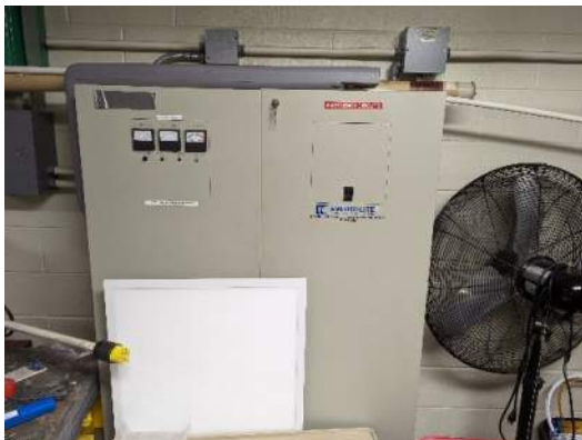
Central Inverter System
