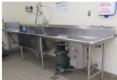
Existing Food Prep and Dishwash Sink without Indirect Drain Connection
