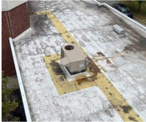
Existing administration rooftop unit
