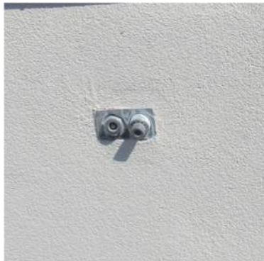
Existing Non-Freeze Wall Hydrant
