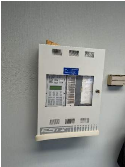
Edwards EST2 fire alarm control panel
