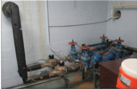
Existing Domestic Water Service
