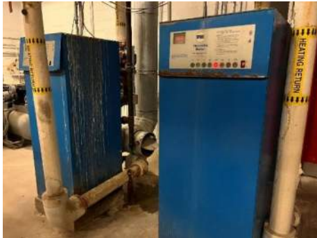
Existing Patterson-Kelley "Boiler Room" Boilers
