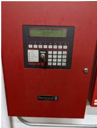
Gamewell fire alarm control panel
