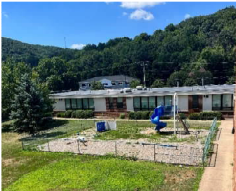
Cracks and damage at hard play area
