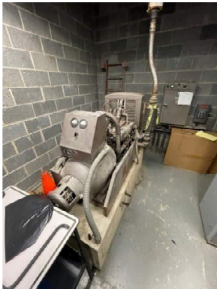
Old abandoned 20KW interior gasoline generator
