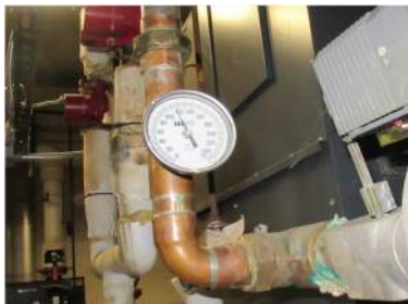
Existing Domestic Water Heater and Observed Corrosion
