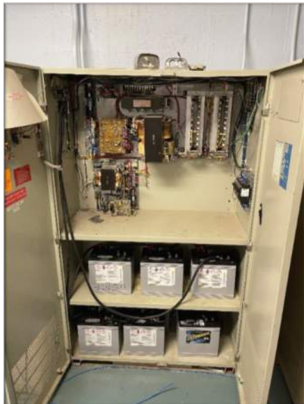
Emergi-Lite inverter for emergency lighting
