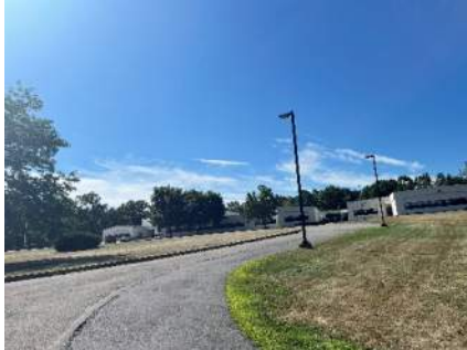
Cracks in drive to main lot
