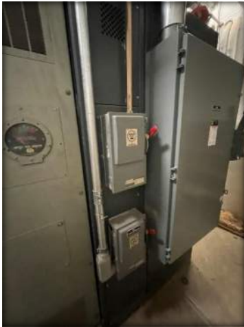
Bus taps on 2000A 480/277V G.E. Switchboard
