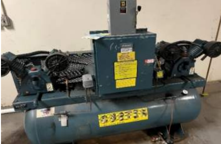
Existing air compressor serving pneumatic control systems
