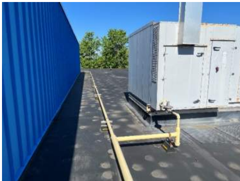
Natural gas piping across roof to packaged rooftop air handling unit
