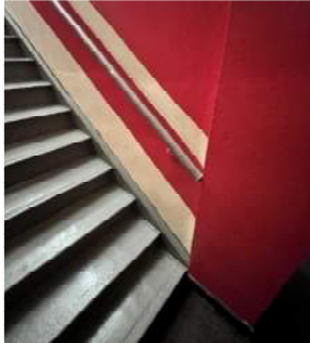
Handrail at stair with no extension
