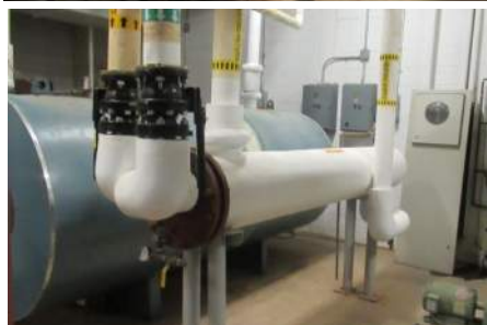
Existing Main Building Domestic Water Heater
