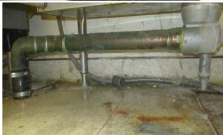
Existing Dishwash Sink without Indirect Drain Connection and Corroded Floor Sink
