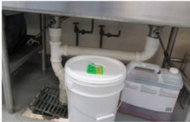
Existing Dishwash Sink without Indirect Drain Connection and Corroded Floor Sink
