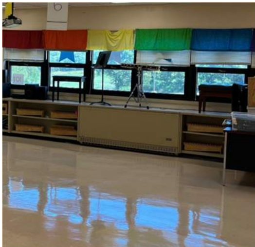
Existing under-window vertical unit ventilator
