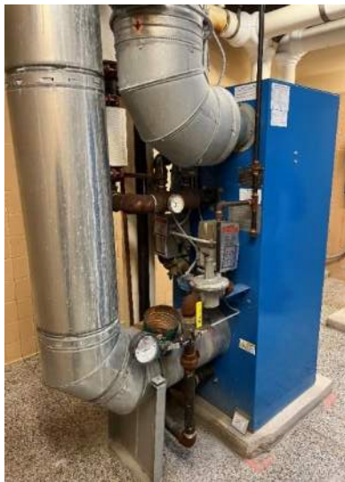
Existing Patterson-Kelley "Toilet Room" Boilers
