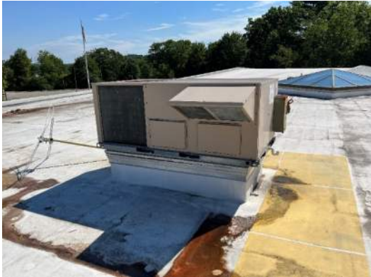
Existing packaged rooftop unit
