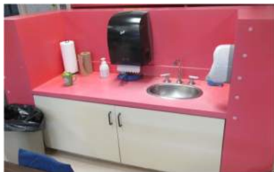
Existing Non-ADA Classroom Toilet Rooms
