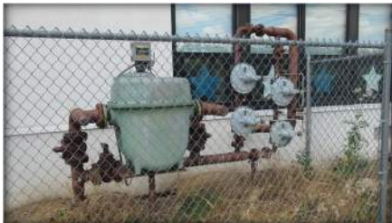
Existing Natural Gas Service
