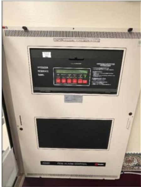
Simplex 4020 fire alarm control panel
