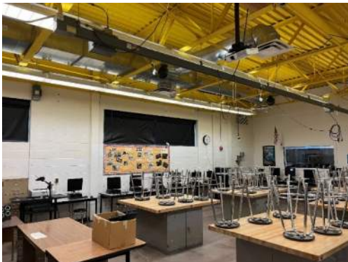
STEM Room with exposed ductwork (Typical for Tech-Ed Wing)
