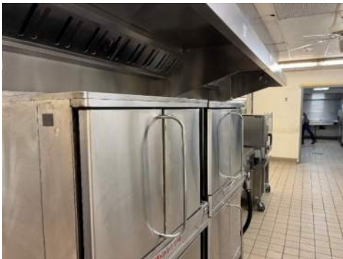
Kitchen grease hood with limited ANSUL system coverage
