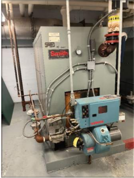
Existing H.B. Smith cast-iron natural gas boiler with Webster burner
