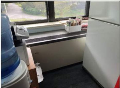
Existing under-window unit ventilator
