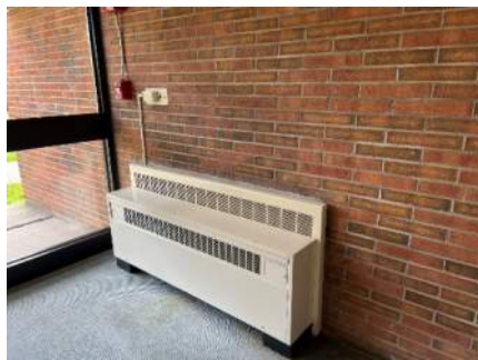
Existing convector/cabinet heater with cabinet heater overlay
