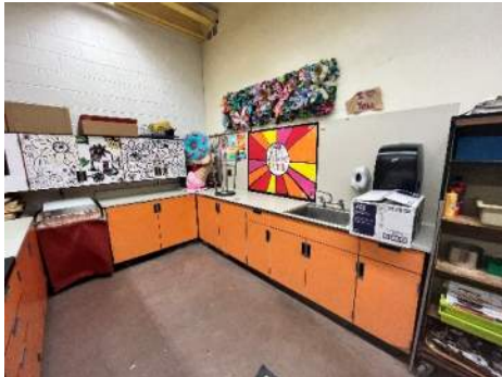
Non-compliant classroom sink in casework
