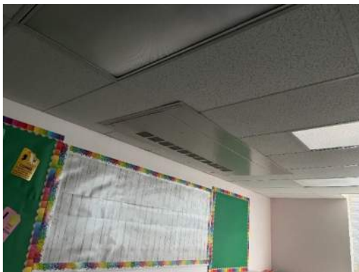
Existing ceiling-mounted horizontal unit ventilator
