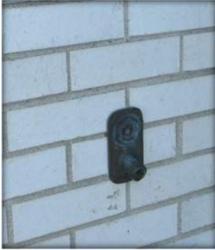
Existing Non-Freeze Wall Hydrant
