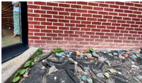
Some cracked mortar and brick staining at courtyard
