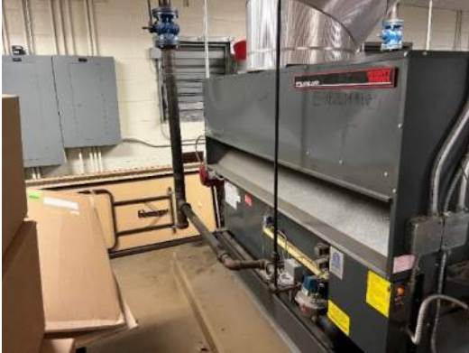
Existing Lars Teledyne cast-iron natural gas boiler
