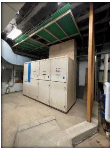
Existing medium voltage switchgear
