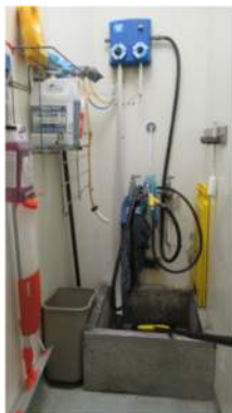
Existing Janitor Service Sinks
