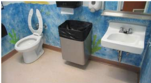
Existing Plumbing Fixtures in Classroom Toilet Rooms
