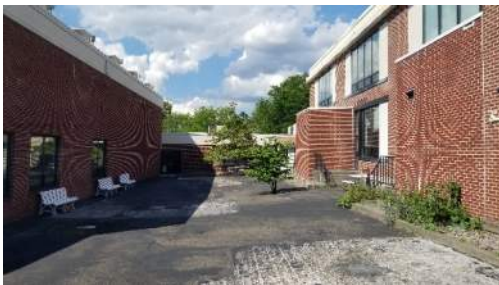
Paving damage at courtyard
