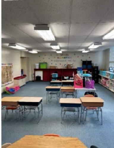
Surface mounted wrap around fixtures
