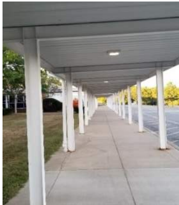
Surface cracking at main entry sidewalk
