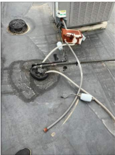
Existing pipe portal and electrical disconnect for the Library Condensing Unit
