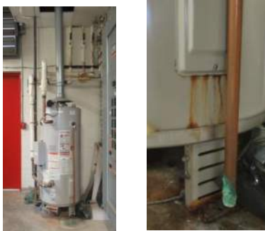
Existing Domestic Water Heater and Observed Leak
