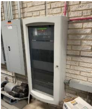
Simplex 4100ES fire alarm control panel
