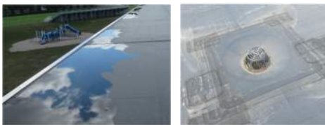
Existing Roof Drain and Ponding at Roof Edge
