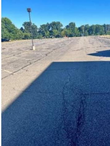
Cracking in staff parking lot
