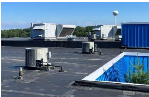
Existing rooftop units and condensing units serving split-DX cooling coils.
