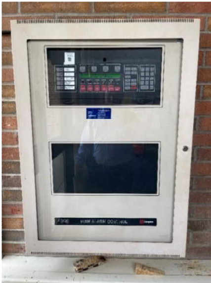
Simplex 4020 fire alarm control panel
