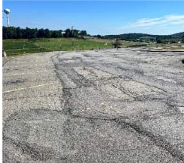
Deteriorating asphalt paving at parking and drives
