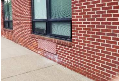
Exterior brick with some efflorescence at openings
