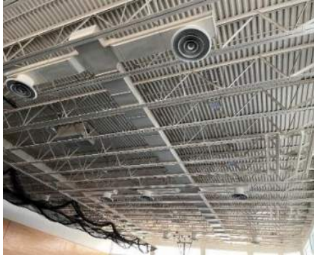
Auxiliary gymnasium supply air ductwork distribution
