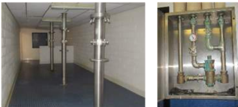
Existing Locker Room Plumbing Fixtures
