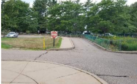
Cracking on driveways
