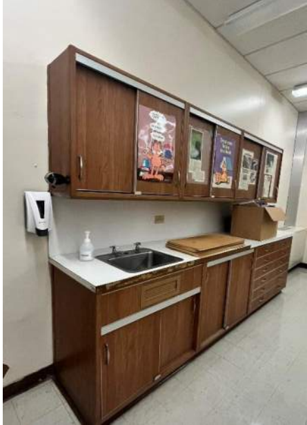
Non-compliant classroom sink fixture
