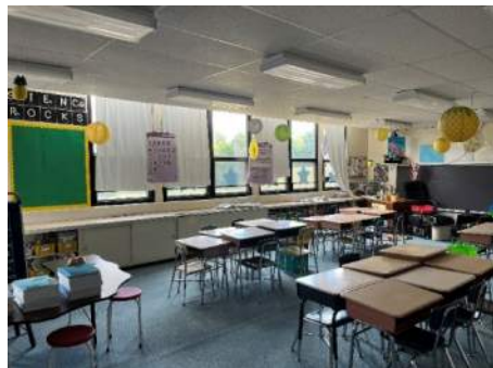
Typical existing Classroom with under-window vertical Unit Ventilator
