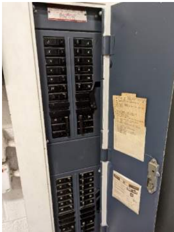
Typical branch distribution panelboard
