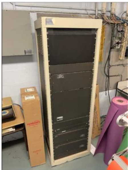
Existing Dukane floor mounted PA rack
