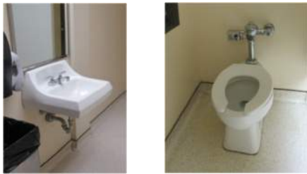
Existing Gang Toilet Plumbing Fixtures
