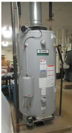
Existing Domestic Water Heater
