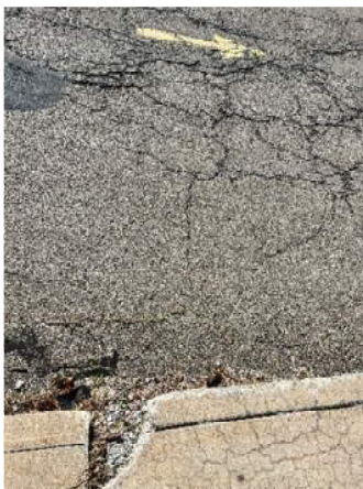
Damaged sidewalk/curb with exposed rebar; asphalt cracking at drive
