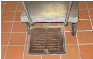
Food Prep Sink without Indirect Drain Connection and Corroded Floor Sink
