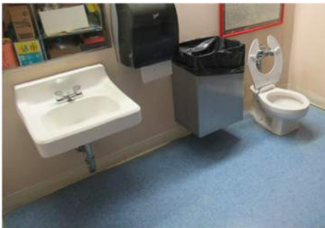
Existing Plumbing Fixtures in Classroom Toilet Rooms
