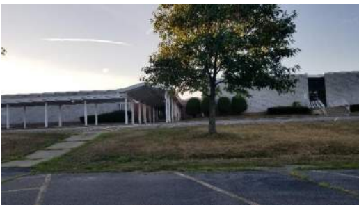
Cracked paving at front entry; steep sloping sidewalk with no handrails; vegetation growth between sidewalk joints
