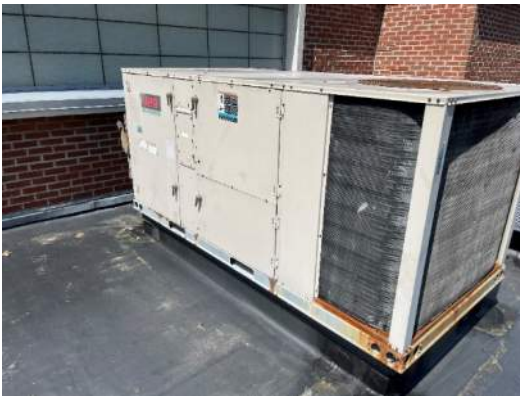
Existing packaged rooftop unit (DX cooling & gas furnace)
