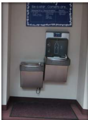
Existing Electric Water Coolers
