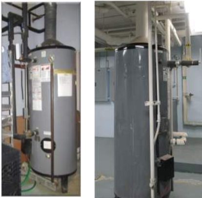
Existing kitchen (left) and main building domestic water heaters
