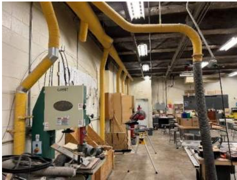
Technical education lab with dust collector array
