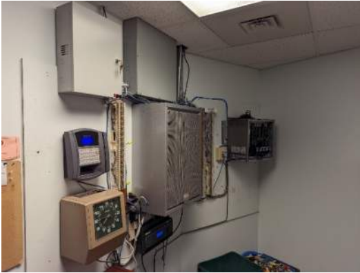
Existing wall mounted PA rack
