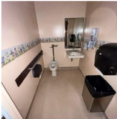
Non-ADA compliant toilet room
