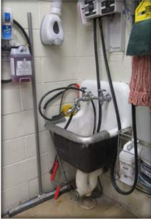
Existing Janitor Service Sink
