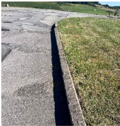
Failing curbs at drives
