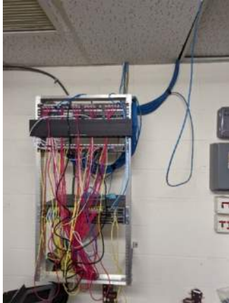
Typical wall mounted data rack
