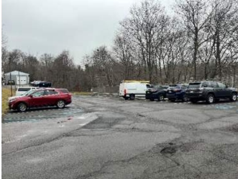
Cracked paving at front entry
