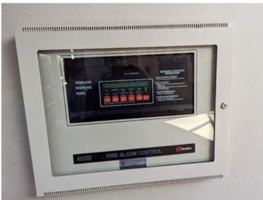
Simplex 4020 fire alarm control panel
