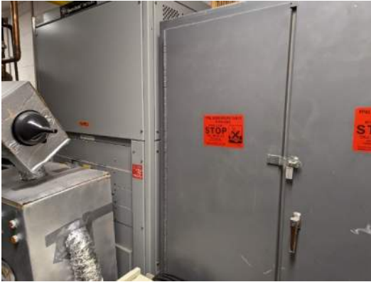
Main Distribution Panel with storage in front
