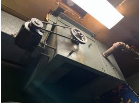
Existing Locker Room H&V Unit (pre-1998)
