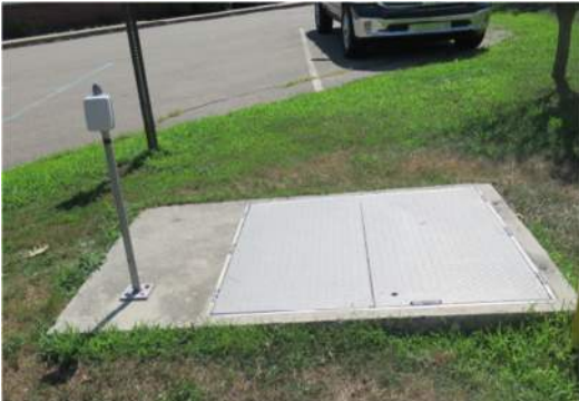
Existing Domestic Water Service Meter Vault
