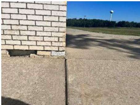
Missing brick, exposing board insulation beyond
