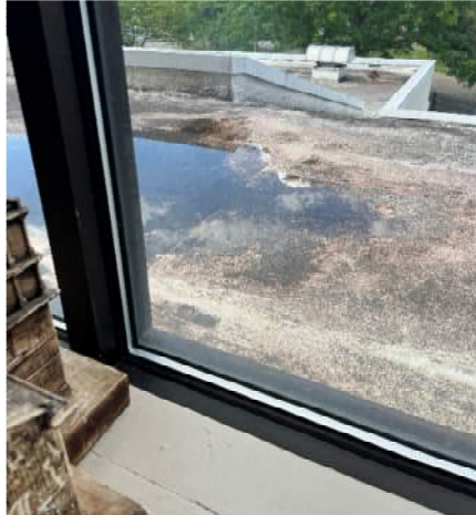
Ponding on toilet room additions
