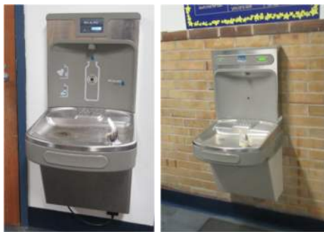
Existing Electric Water Coolers
