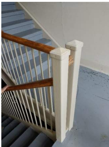
Guardrail that is too low; missing handrail
