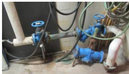
Existing Domestic Water Service
