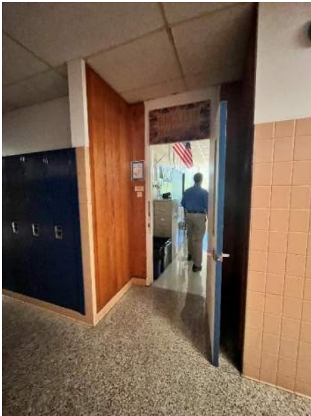
Classroom entry without compliant door clearance
