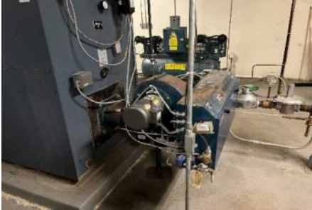
Existing Weil Mclain cast-iron dual fuel boiler with Power Flame burner
