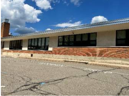
Cracks and damage at drives/parking
