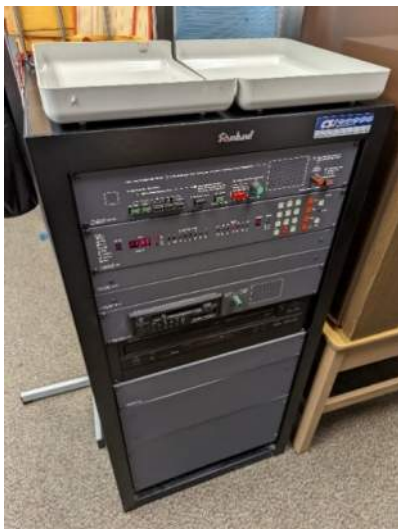
Existing PA rack
