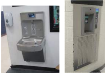
Existing Electric Water Coolers
