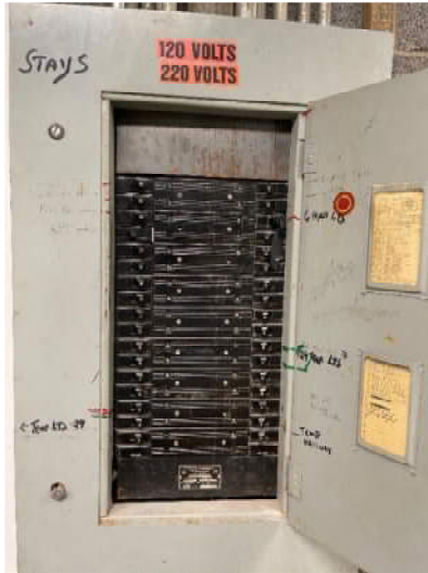
Old Westinghouse panelboard
