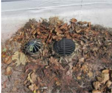
Existing Roof Drain and Ponding at Roof Edge
