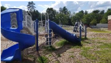
Cracks and damage at hard play area
