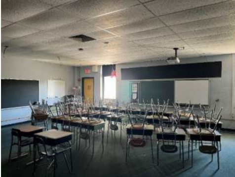
Pod classroom with single supply air diffuser.
