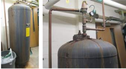
Existing Domestic Water Heater Expansion Tank and Observed Leak
