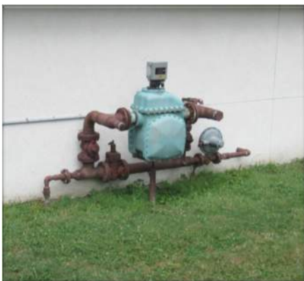
Existing Natural Gas Service/Meter
