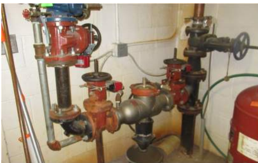
Existing Fire Protection/ Domestic Water Service Entrance
