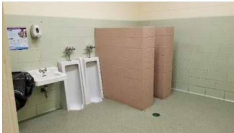
Non-compliant toilet room in locker area
