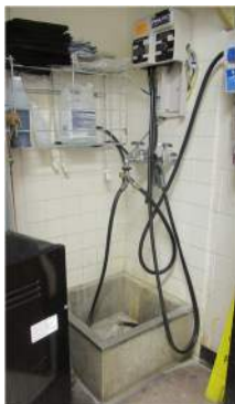
Existing Janitor Service Sinks
