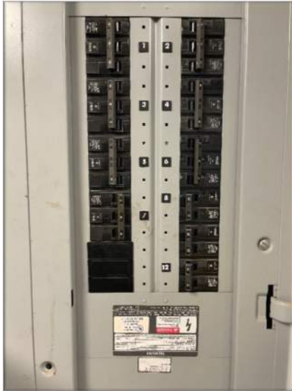
Typical Siemens 1995 branch distribution panelboard
