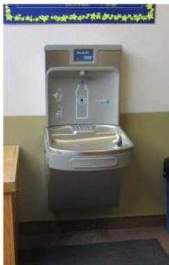
Existing Electric Water Coolers
