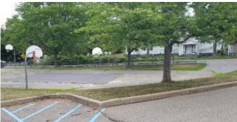
Hard play with cracking/large patches
