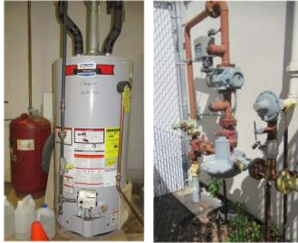
Existing Domestic Water Heater and Gas Service
