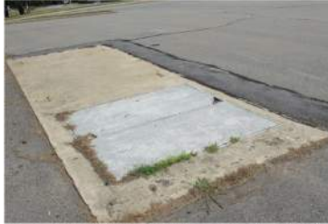
Existing Domestic Water Service Meter Pit
