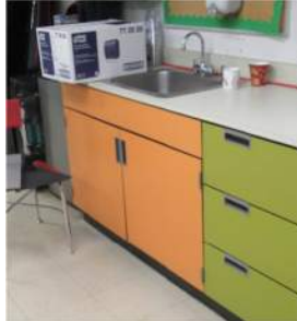
Existing Non-ADA Sinks
