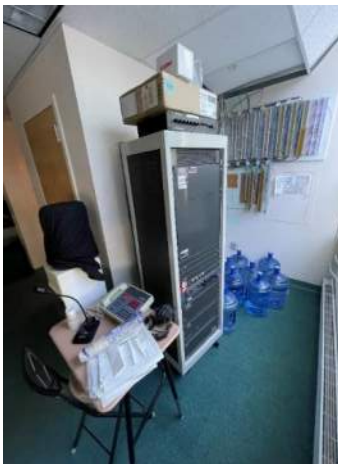
Existing PA rack on wheels
